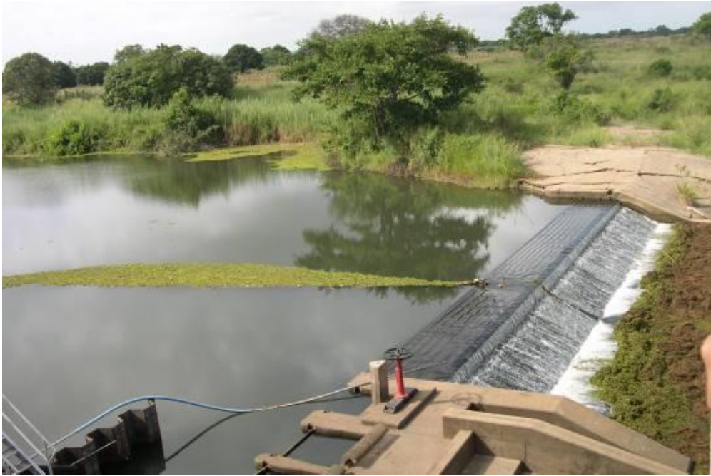
Figure 4: intake for the Umbeluzi water treatment plant that serves Maputo (courtesy of AdeM).
